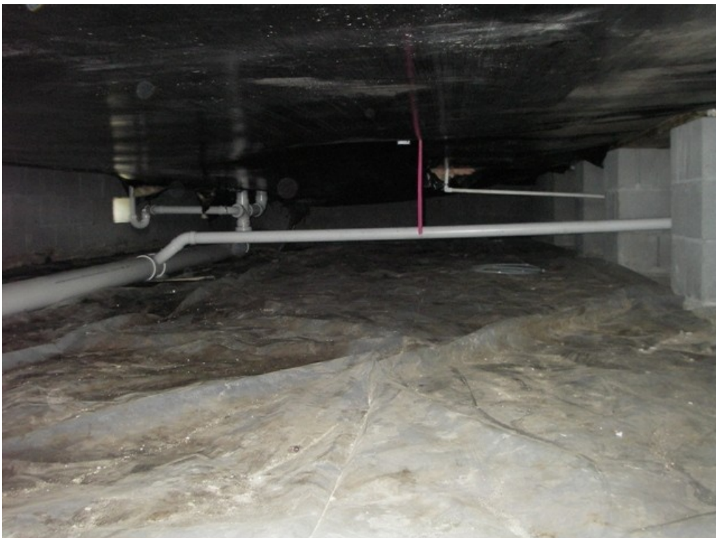
Figure 7. Baton Rouge vented control crawl space.
