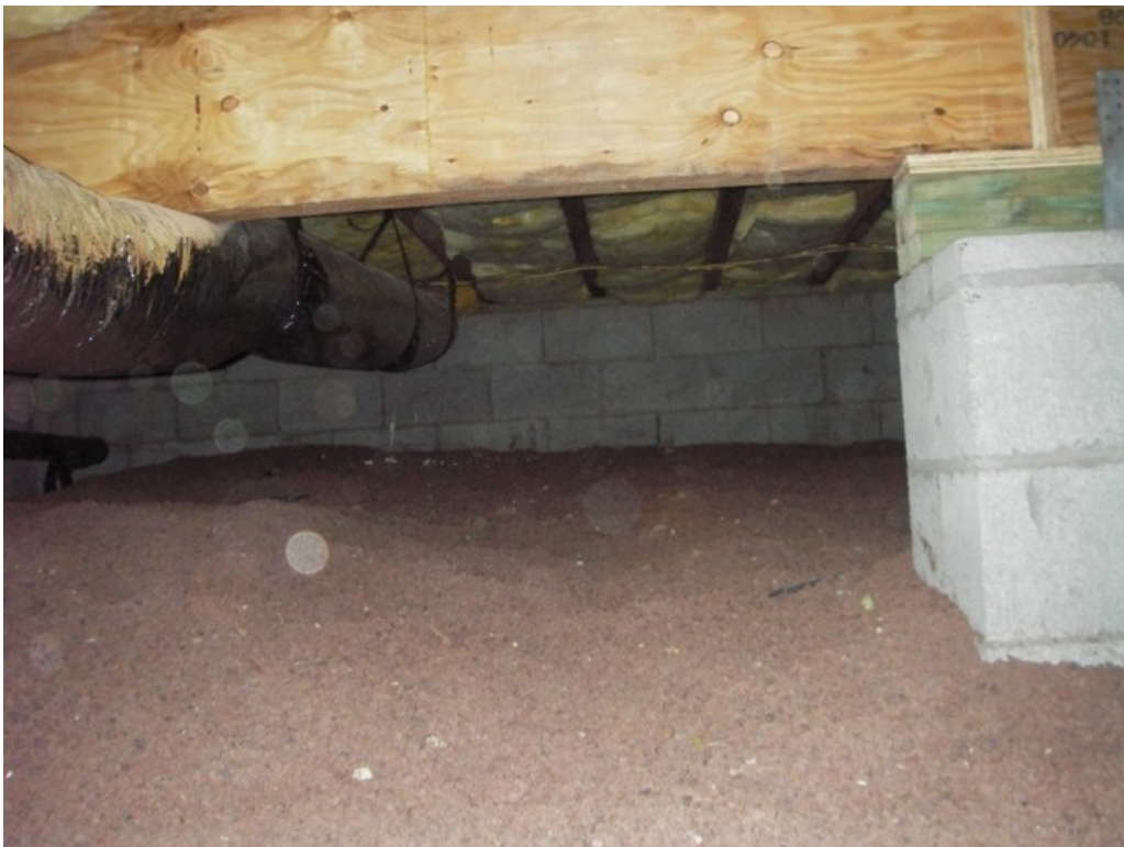
Figure 18. Flagstaff vented crawl space.
