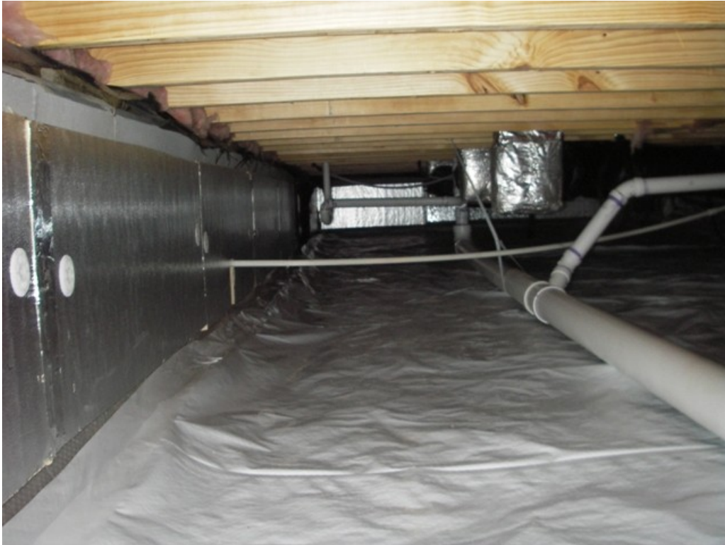
Figure 10. Baton Rouge finished wall-insulated closed crawl space.
